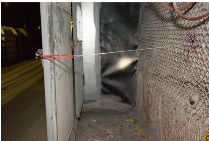
Air Lock Doors Wired Open
