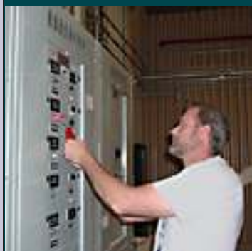
Paul Orr (WTS) performs a lockout/tagout procedure on the TRUPACT maintenance facility electrical panel.
