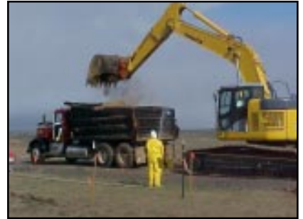
Workers remove overburden soil from the designated retrieval area of Pit 4 at INEEL's Subsurface Disposal Area.
