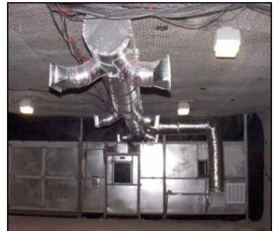
The underground lunchroom features better air conditioning and more lighting. Photos courtesy of Melody Smith, WTS
