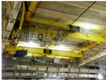
The addition of two cranes increases waste handling reliability.
