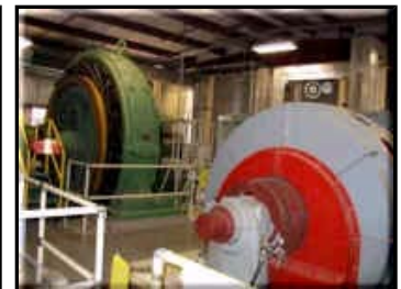
Hoist motor (green) and synchronous motor generator
