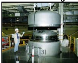
RCT swipes the inside of the OCV lid.
