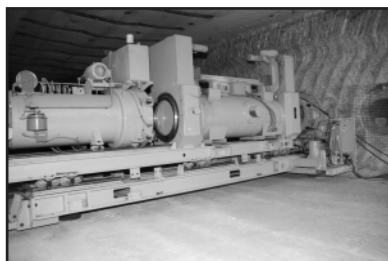
RH-TRU waste is disposed in the walls of the disposal rooms using shielded horizontal emplacement equipment.
