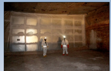
Panel 7, Room 7, exhaust side closure
