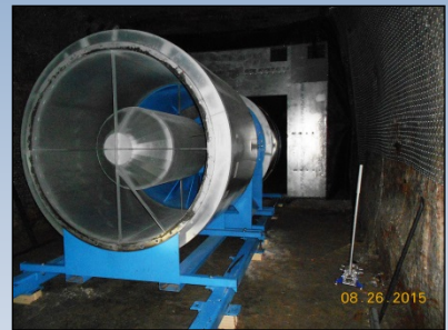
Supplemental Ventilation System fan installed in the S90 drift
