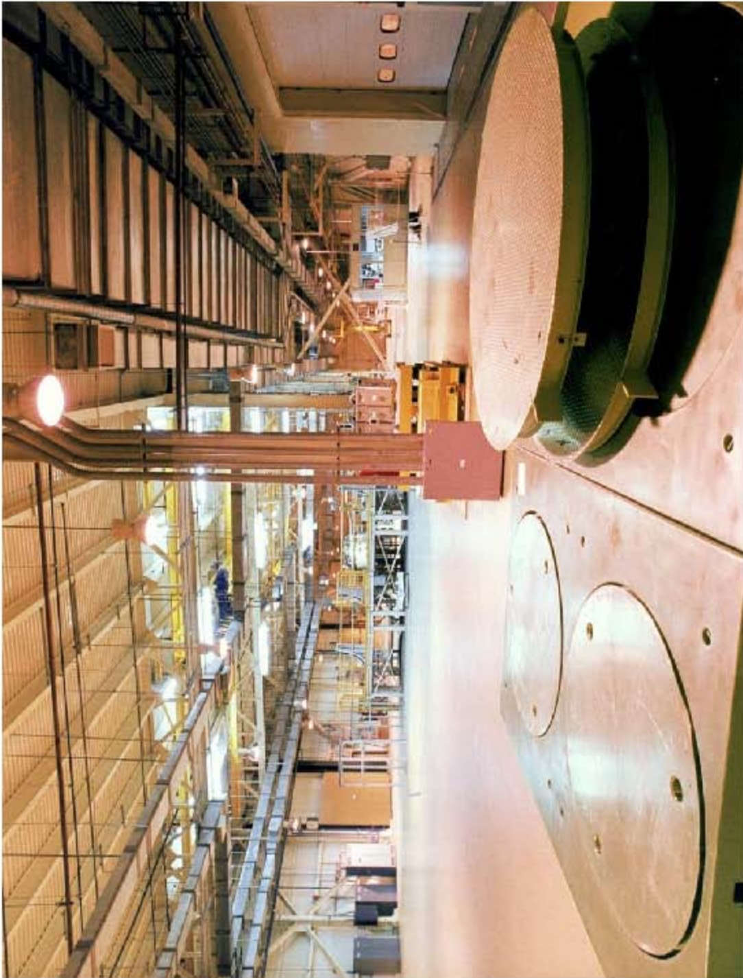
Figure O4-6 Westward View of CH Bay of the Waste Handling Building
