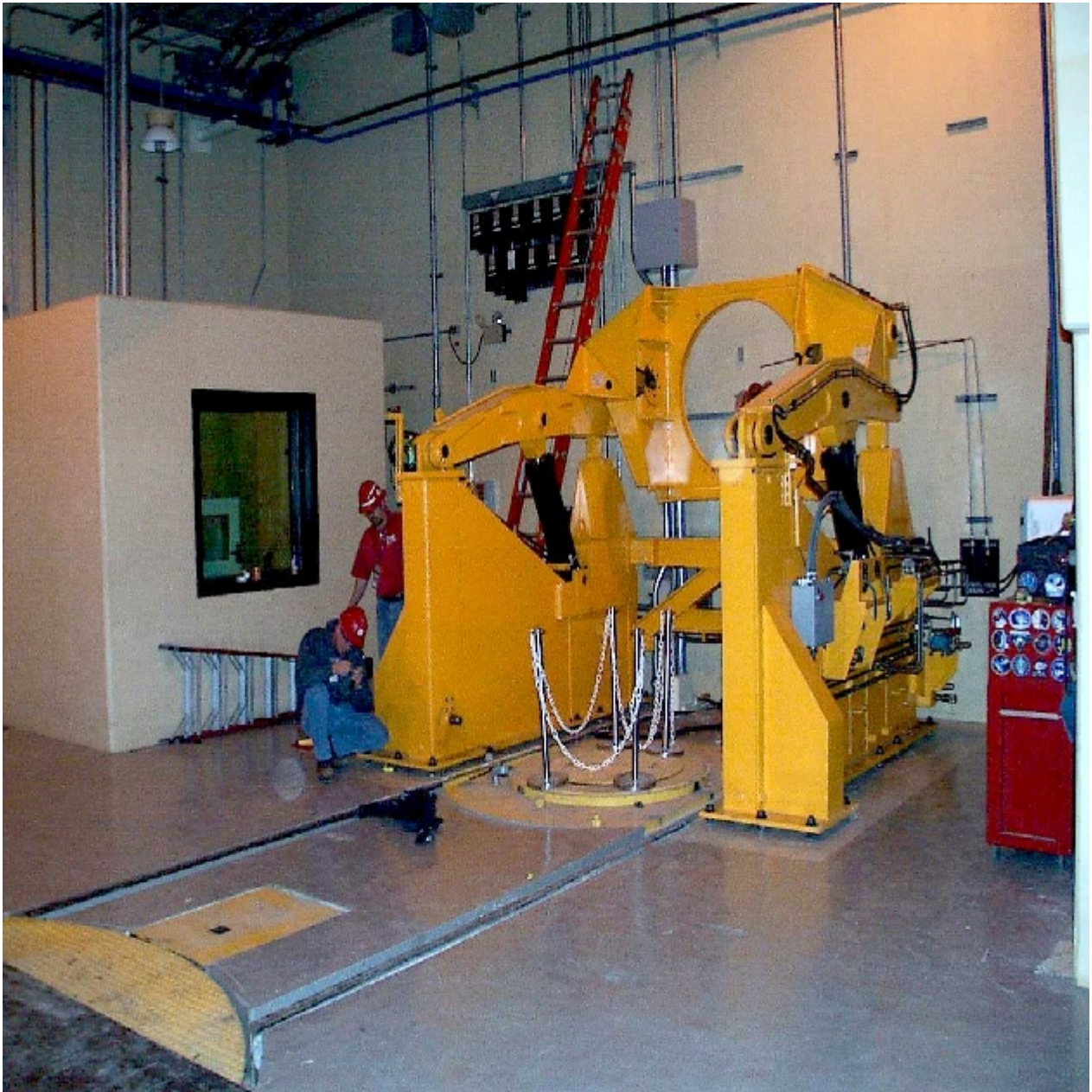
Figure O4-12 Facility Cask Loading Room and Facility Cask Rotating Device
