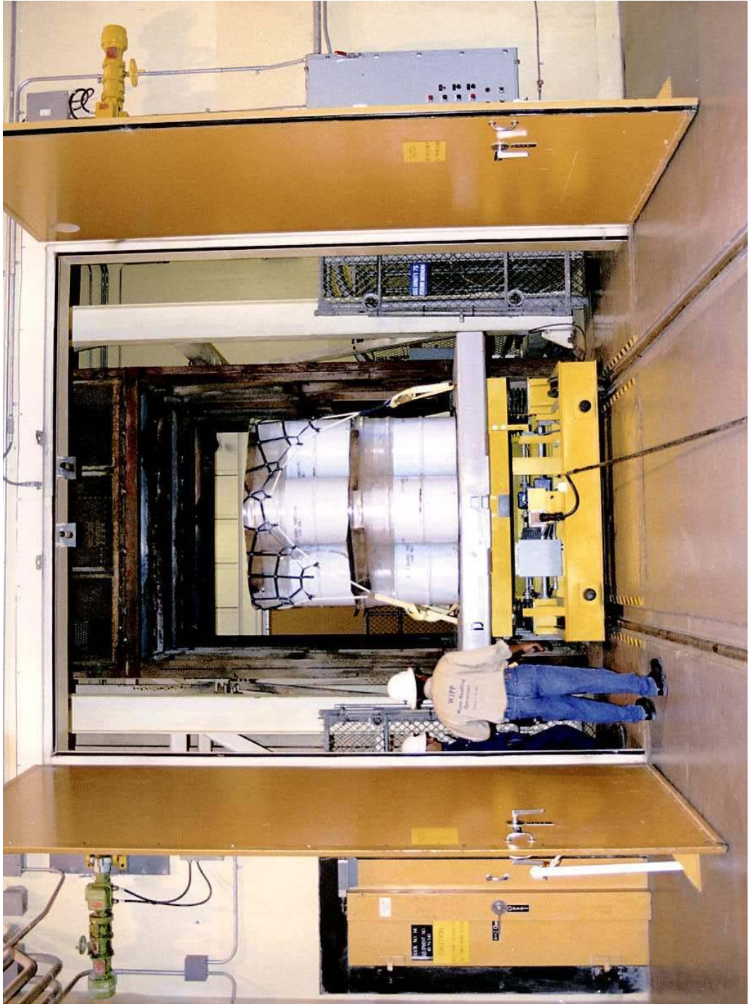
Figure O4-7 Waste Shaft Conveyance - Loading Facility Pallet with CH Waste, Waste Handling Building
